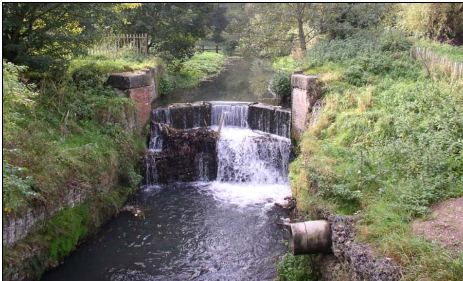
Photograph 4.6 - Keddington Church Lock – Note gates have been removed
