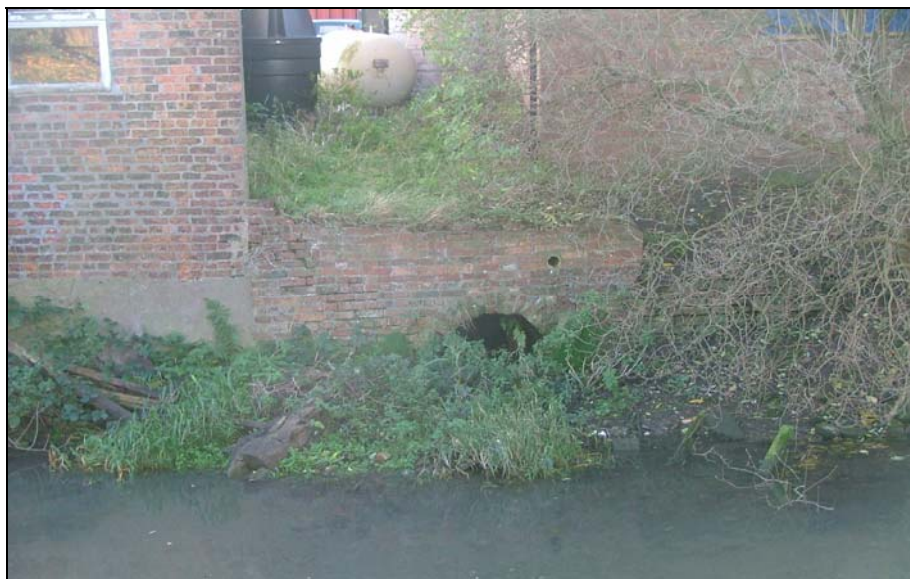
Photograph 2.1 - Inlet culvert from River Lud to Louth Canal at Riverhead (now abandoned)
