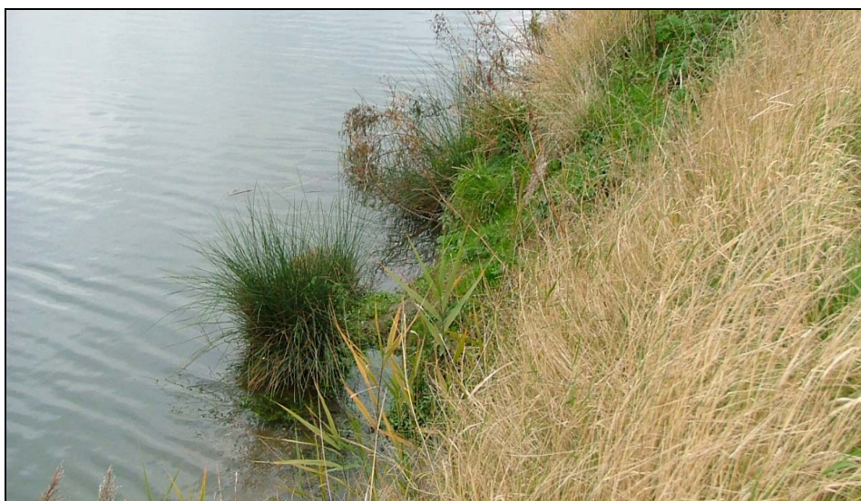
Photograph 3.4 - Bank erosion downstream of Fulstow Footbridge
