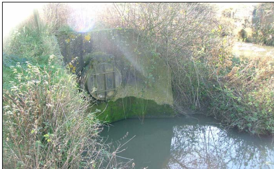
Photograph 8.3 - Outfall from Great Eau Raw Water Transfer Main
