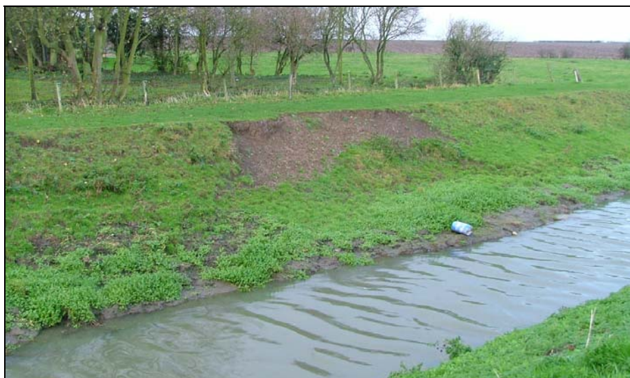
Photograph 3.1 - Bank Slip downstream of Alvingham Canal Church Footbridge
