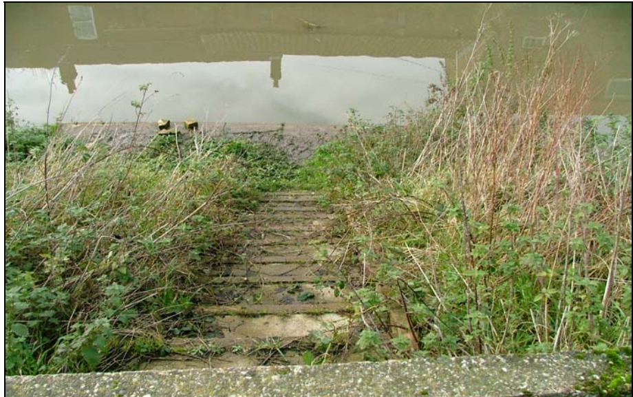
Photograph 3.7 - Derelict concrete landing stage/steps upstream of Austen Fen Bridge
