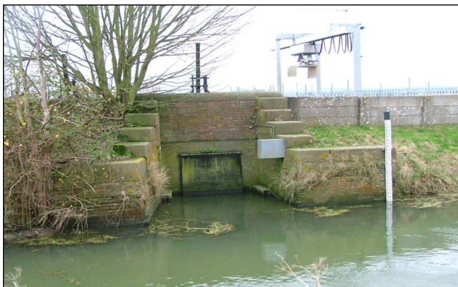
Photograph 8.5 - Outfall from Lindsey Marsh Drainage Board Thoresby Bridge Pumping Station
