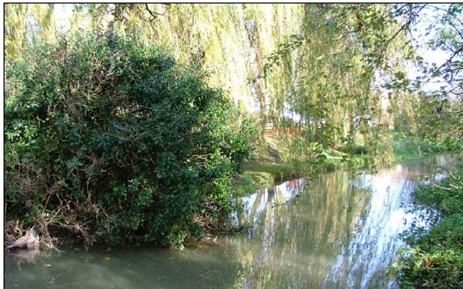
Photograph 3.3 - Overhanging trees between Top Lock and Keddington Church Lock and erosion of bank toe
