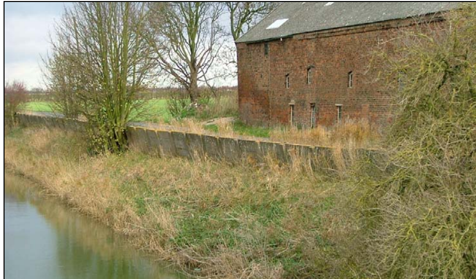
Photograph 3.2 - Leaning wall downstream of Fire Beacon Bridge
